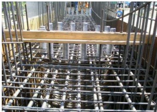
Figure 2.30 Corrugated ducts in precast cap beam in Washington State. (Kapur, et al., 2012)
