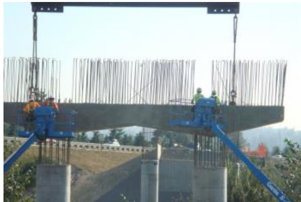
Figure 2.31 Placement of cap beam on column bars inserted in corrugated ducts in Washington State. (Kapur, et al., 2012)
