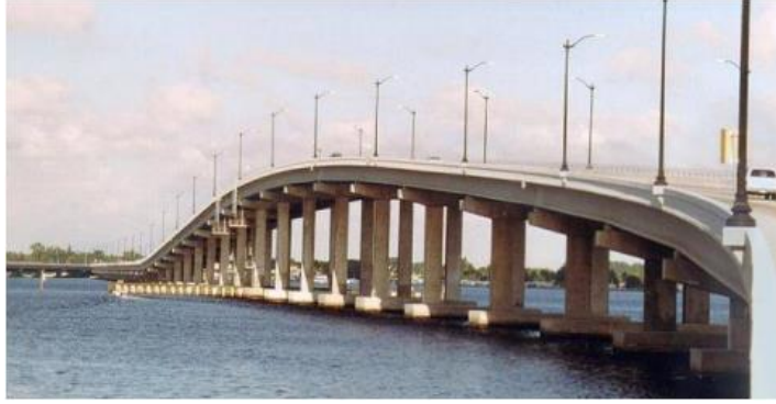
Figure 2.10 Precast open frame pier bent constructed bridge in Florida. (Culmo M. P., 2011)
