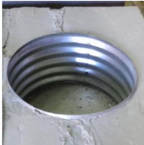
Figure 2.50 CMP void in pile cap. (Hosteng, Phares, & Redd, 2016)
