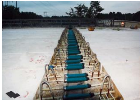
Figure 2.37 Grouted coupler as continuity splice over pier in Massachusetts. (Kapur, et al., 2012)
