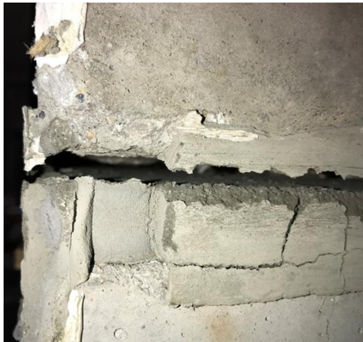
Figure 5.19 GRBC rear face crack due to vertical load.
