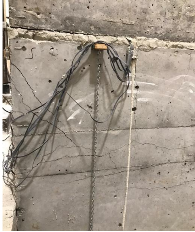
Figure 5.24 Pile coupler pile cap cracking due to vertical load.
