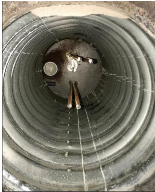
Figure 4.48 Bottom view of CMP void.
