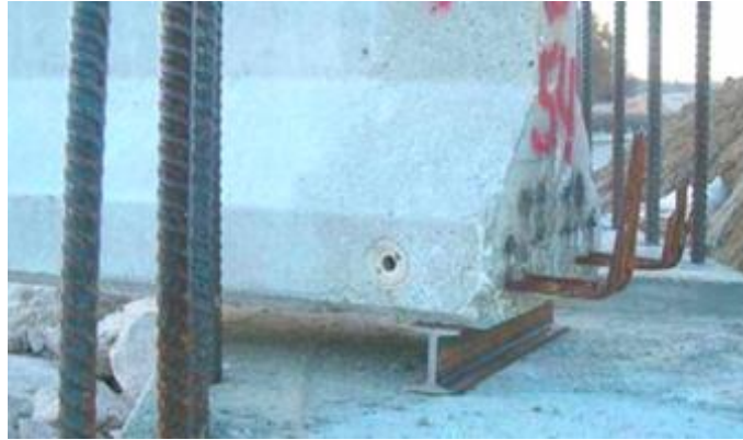
Figure 2.23 Beam end supported by abutment cap by steel beam to provide clearance for concrete placement. (Wipf, Klaiber, & Hockerman, 2009)
