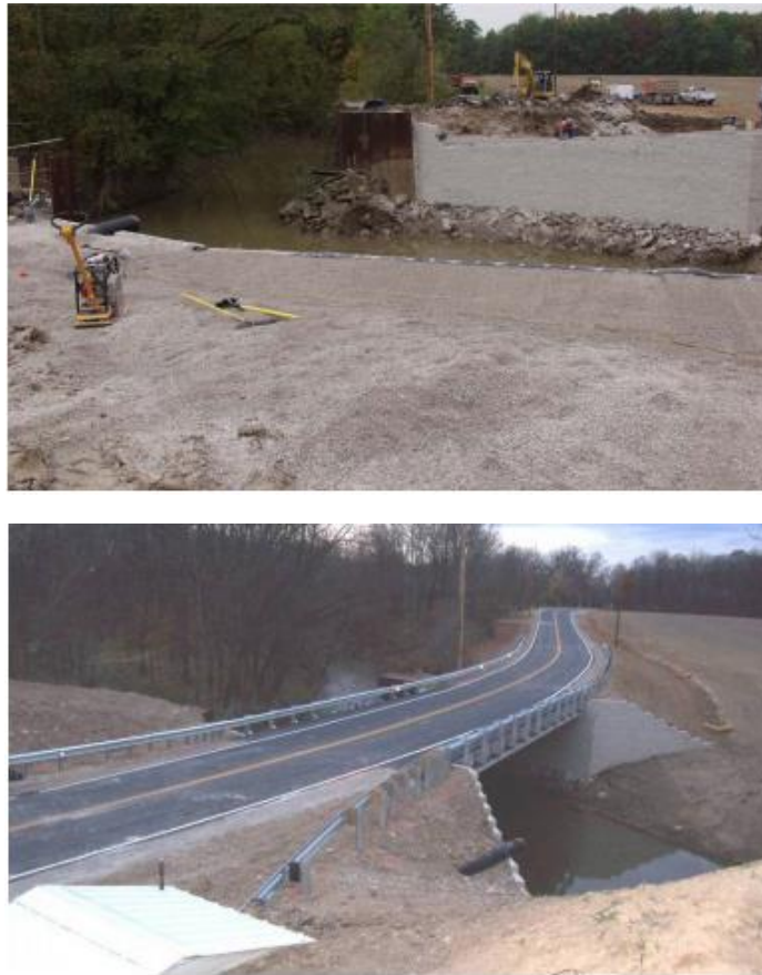
Figure 2.4 GRS-IBS bridge in Ohio. GRS Abutment during construction (top). Completed bridge built in 47 days (bottom). (Culmo M. P., 2011)
