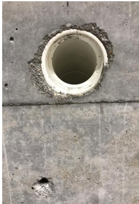
Figure 4.53 Surfaced 3 in. duct and 1 in. duct found after chipping concrete.
