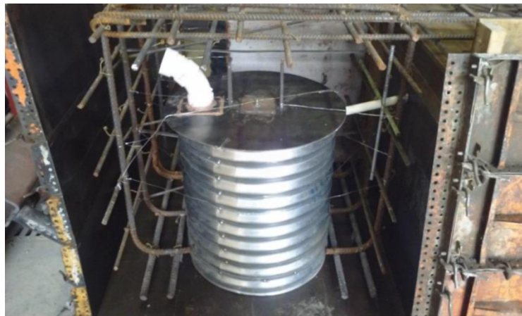
Figure 2.48 Side view of CMP void. (Hosteng, Phares, & Redd, 2016)
